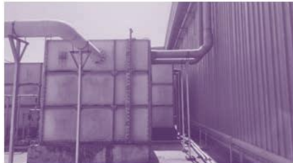
Rainwater harvesting system – Kianjoo Can (Myanmar) Company Limited
