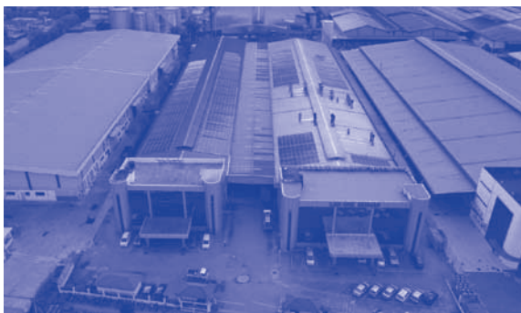
623 kWp solar system at Aik Joo Can Factory Sdn. Berhad Lot 2244
