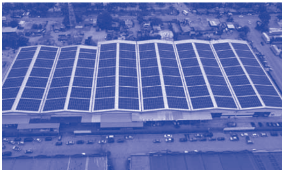
2,137 kWp solar system at KJCF plant in Batu Caves
